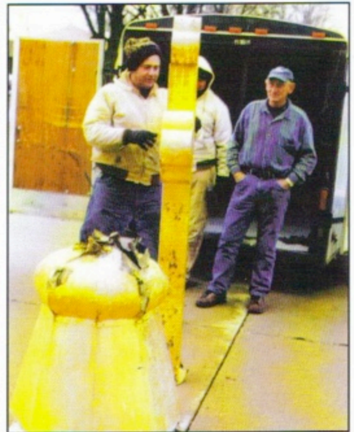
In December 2003, strong winds broke the original king pin and damaged the base of the six-foot cross which graces the top of the steeple. It was repaired and returned in April 2004.
